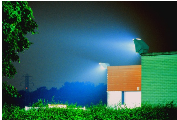
Figure 3.1 - Two identical metal-halide throw lights are shown here having dissimilar up-light. This is largely achieved by the installer using an incorrect tilt angle for one of the luminaires.
